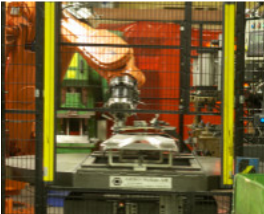
Two automatic resistance welding machines operated by ABB robots. One of them equipped with Vision System.
